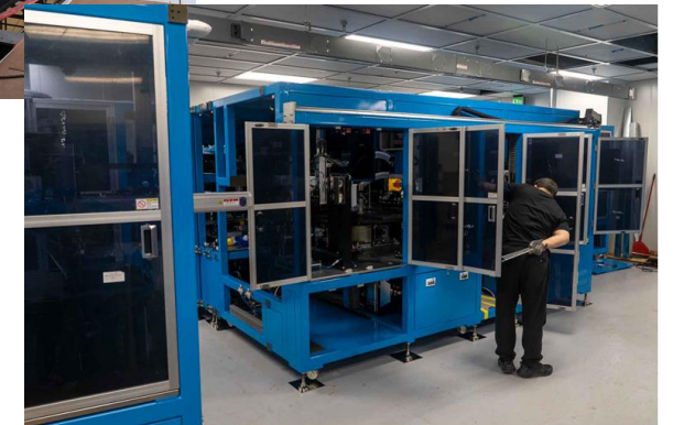
From top to bottom: EV line dehumidifier being lowered into Solid Power building, installation of EV line dehumidifier, start of installation of automated cell manufacturing equipment
